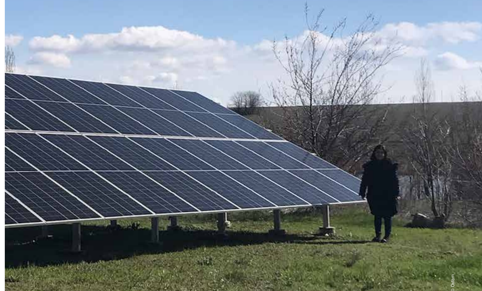
Solar panels to power a well constructed by Oxfam in Yuzhne, Ukraine.
