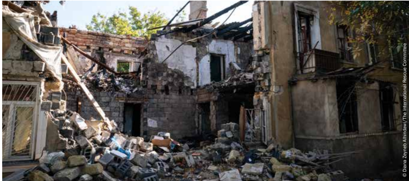
Residential buildings that were heavily damaged during a missile attack in Mykolaiv, Ukraine.
