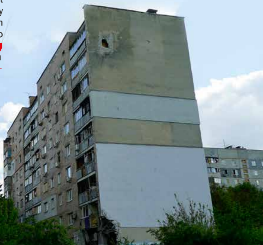
A damaged high-rise building in Kharkiv, Ukraine's second-largest city where DEC member charities are providing essential aid to people sheltering in basements and bomb shelters
